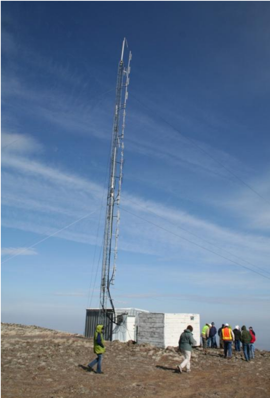
Figure A.18. Columbia Communications Tower (Locale 6). Photo taken at 345 degrees on 3/19/09 by Doug McFarland.
